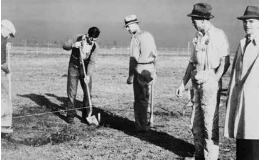
Russell Robinson (right) supervises the first groundbreaking construction at the new NACA Ames Aeronautical Research Laboratory in 1939. (NASA G-325 (0-82))
