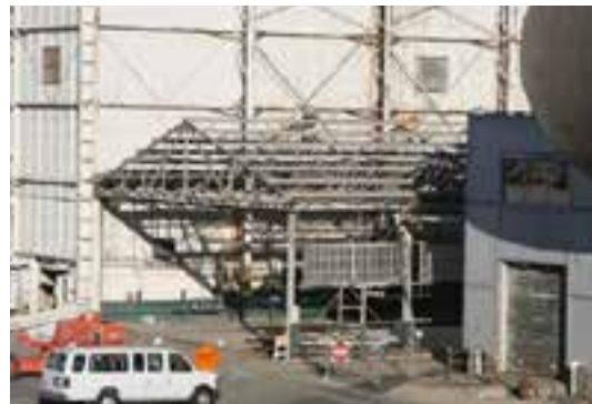
Comparison of a photograph taken during the construction of the Full-Scale Tunnel annex hangar (left) with a photograph showing the hangar during demolition in 2011 (right) shows the structure of the facility after 80 years. (G. Lee Pollard)
