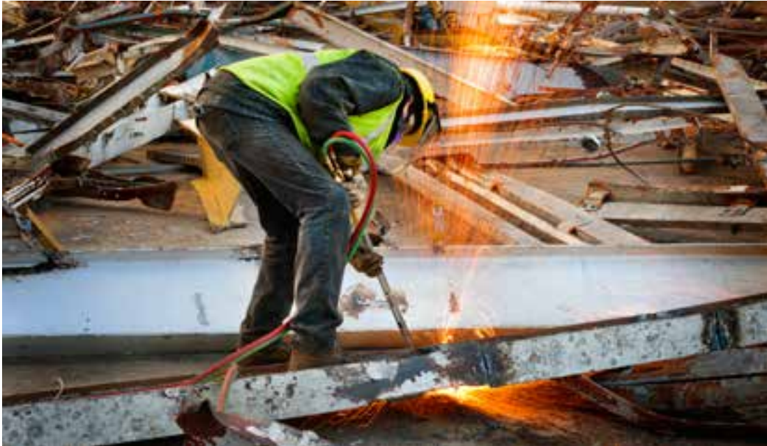
Workmen cutting up exterior structures removed from the Full-Scale Tunnel in January 2011. (NASA 2011-L-00152)
