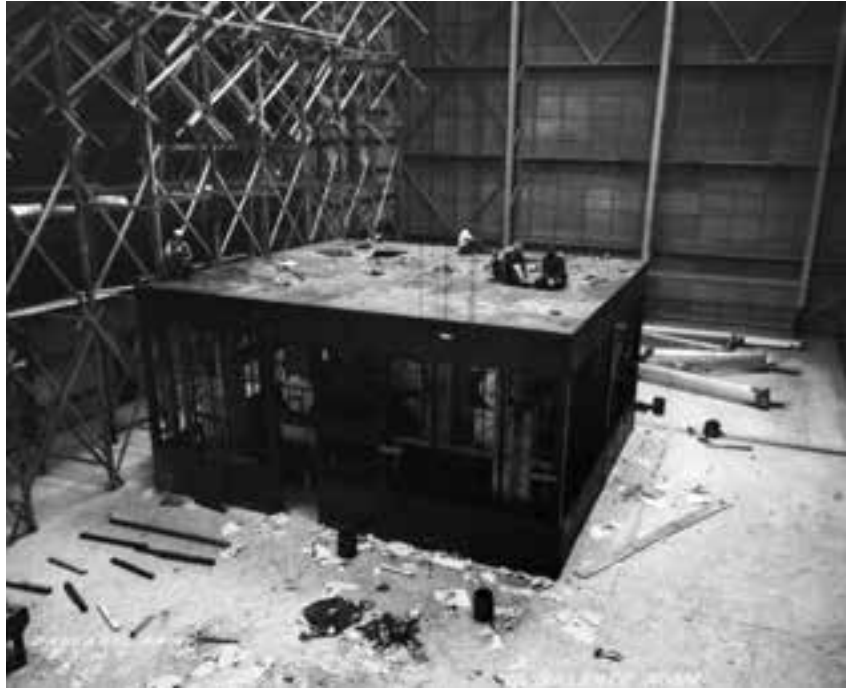
Work to enclose the balance and scale areas was conducted simultaneously with the entrance-cone modifications. (NASA EL-1999-00421)
