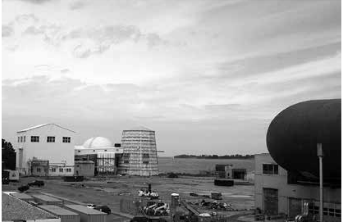
The demolition of the Full-Scale Tunnel was completed in early 2011. This view of the vacant space previously filled by the tunnel was taken in June 2011. The cylindrical building in the center is the Langley 20-ft Spin Tunnel and the tunnel circuit for the Langley 8-ft Transonic Pressure Tunnel is seen at the right. The 8-ft TPT was also demolished in 2011. (Lee Pollard, NASA)
