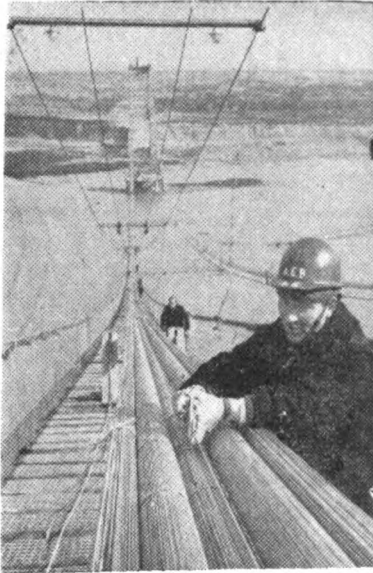
BRITAIN'S NEW SEVERN BRIDGE suspended 400 feet above the River Severn in South west England, a workman makes the suspender cables for the new Severn Bridge which crosses the river between Aust and Beachley. The bridge will be completed in 1966.
