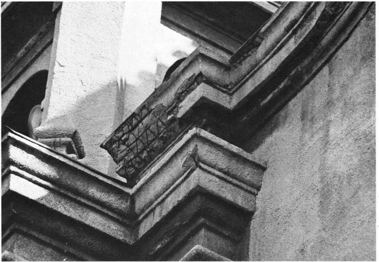
The recent earthquake did more than just superficial damage to Throop; damage to the pre-Field Act structure forced abandonment of the venerable landmark.
