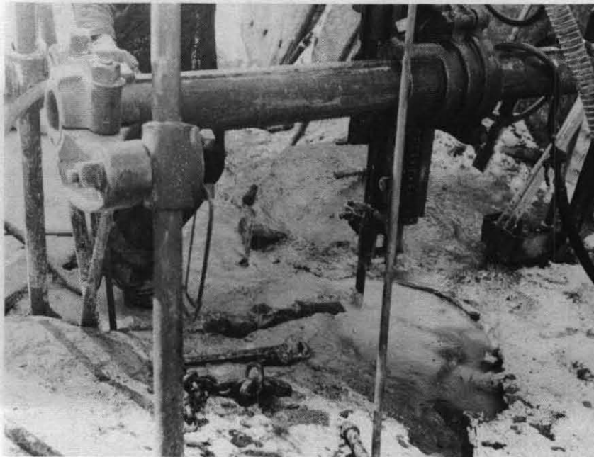
FIGURE 9. Closeup view of leyner bar drilling as practiced since about 1950. Note absence of visible dust as a result of using wet methods.
